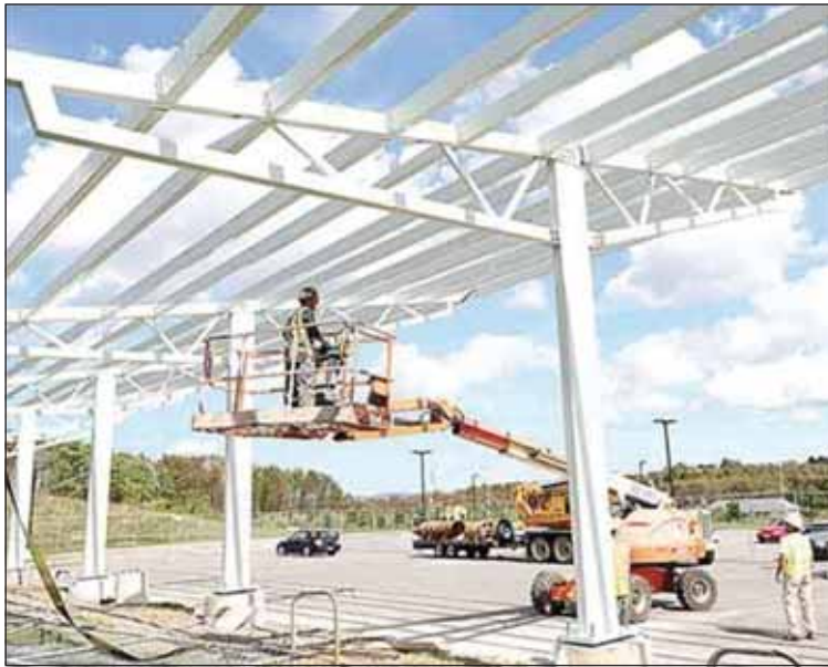
These solar panels, shown when under construction in the parking lots, are still up and running, unlike those atop college buildings.
